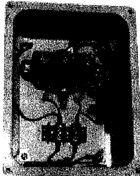
Hose Reel Control Box with Breaker
